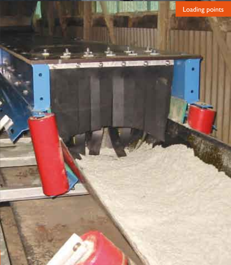
Belt tearing detector
