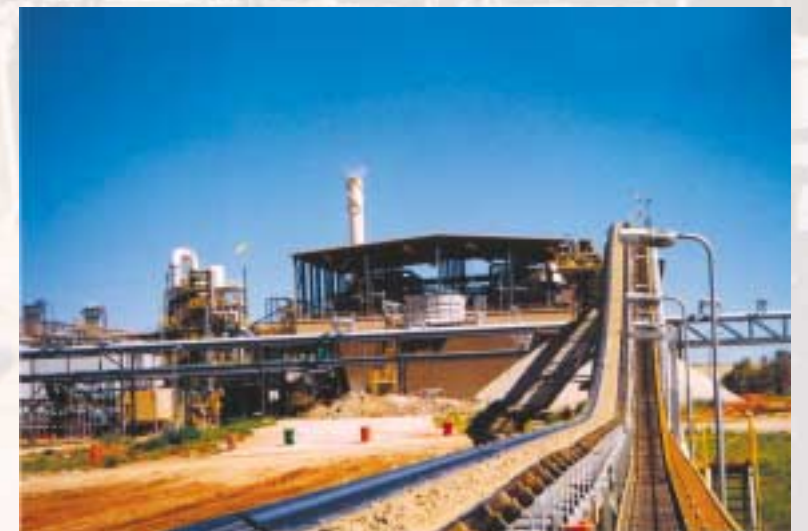
Sun Metals - Zinc Refinery, Zinc Concentrate Conveyors Location: QLD, Australia
