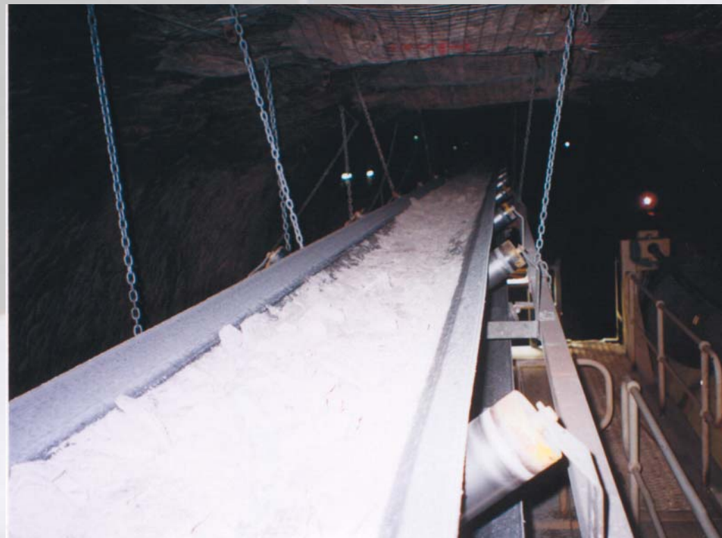
TBM, Spoil Removal Underground Conveyors Capacity: 600 tph, Length: 15,700 m, Location: NSW Australia
